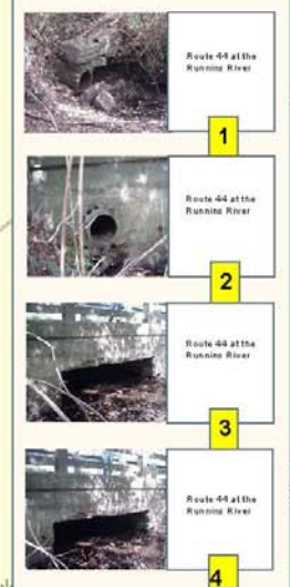
Route 44 at the Running River: there is an 18" concrete pipe in a concrete and stone headwall. The pipe is in good shape. The headwall was collapsed in places and the northern base has eroded in places. The concrete headwall of the bridge over the Running was cracked and weathered in spots. Some erosion at the base is evident. The Running River was low but had a fairly good flow. No silt was clear when observed but a level odor was present.
