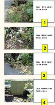
Lava Mitts at Turtle Brook. 5' concrete pipe in stone and cement headwall. Some exposed rebar and part of the lower headwall has collapsed into Turtle Brook. The road surface has sloughed and eroded near this structure. The gravel base is compromised in spots and runoff can drop directly into the waterbody from the road at this point. Turtle Brook had a steady flow but shot of it.
