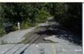
Williams St. Bridge near Robinson Pond. Upgradient is a Priority Habitat area and a Zone II area for a municipal well.
