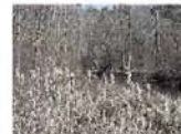
Photo 1 (Photo 1): Sediment and debris at drainage outflow pipe from the Freetown Boat Ramp at Pt. 10.
