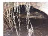
Photo 2 (Photo 2): Drainage outflow pipe at the Freetown Boat Ramp at Pt. 10 into Long Pond.
