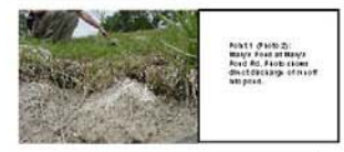
Point 1 (Photo 1): Runoff from 20' wide road into pond. Runoff is directly discharged into the pond buffered by a residential beach area. Condition of roadway is fair to good with a 3 - 8% slope.
