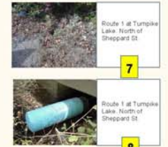
Route 1 at Turple Lake, north of Sheppard St: ⑦ concrete culvert goes under Route 1 and connects waterbodies; asphalt swales on both sides of the road. Slopes greater than 25% to the water. Channelization and erosion occurring. Large plastic tank blocking culvert on the west side. Chunks of asphalt and road reflectors from recent resurfacing are scattered along roadside at the top of the banks behind guard rail. Silt and debris evident below swales on both sides.
