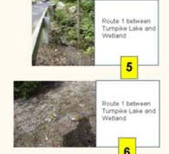
Culvert under Route 1 between Turple Lake and wetland (NW): collapsing silt fence, MHD cones, pavement chips and debris remain from resurfacing. New asphalt swale, >35% slope to the headwall. Some debris and very heavy silt at the base of the swale. On both sides of Route 1, there is so much silt coming off the road that silt fences have collapsed in spots and debris is accumulating around the banks. Flow attenuators should be considered.
