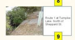
⑨ Site without a photo located at West Bacon (Rte 6) at the Plainville Cemetery. No reveal left to the curbing on the roadway, allowing runoff to go directly into the brook off of the bridge. A cold water fishery is upstream from this site.
