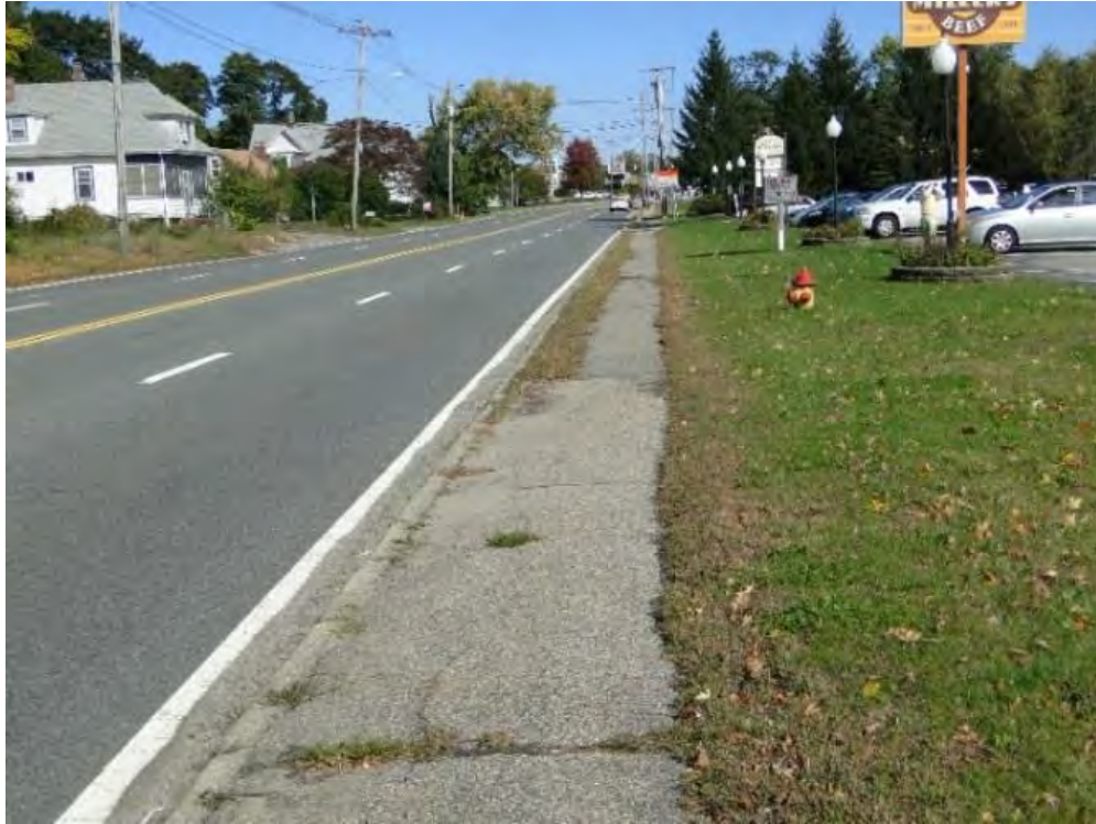
Figure 5: Poor sidewalk conditions on Route 1A south of Route 123
