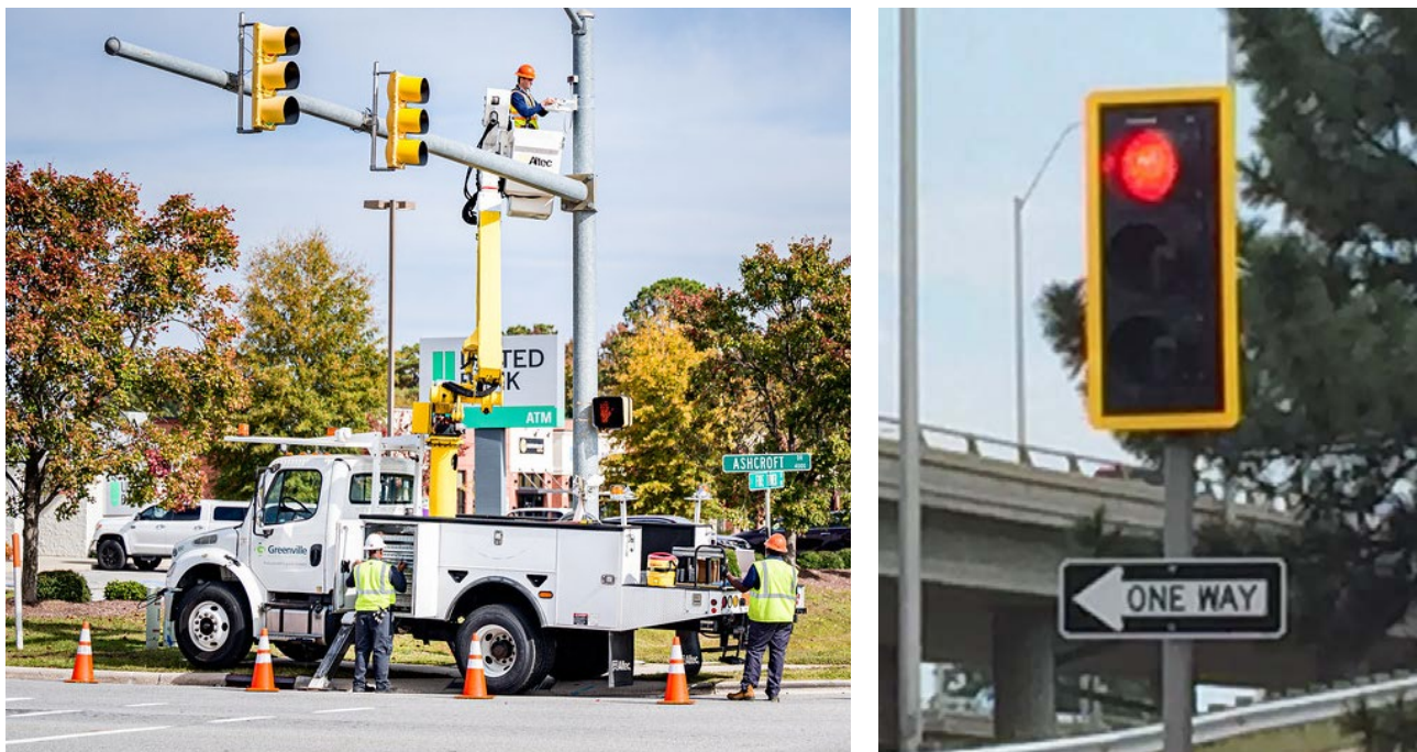
Figure 4-10: Workers updating signal equipment and a signal head with a retroreflective backplate.
