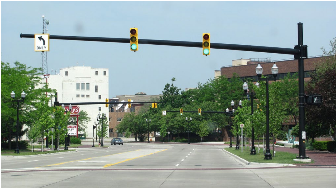
Figure 4-15: Signal Mast Arms
