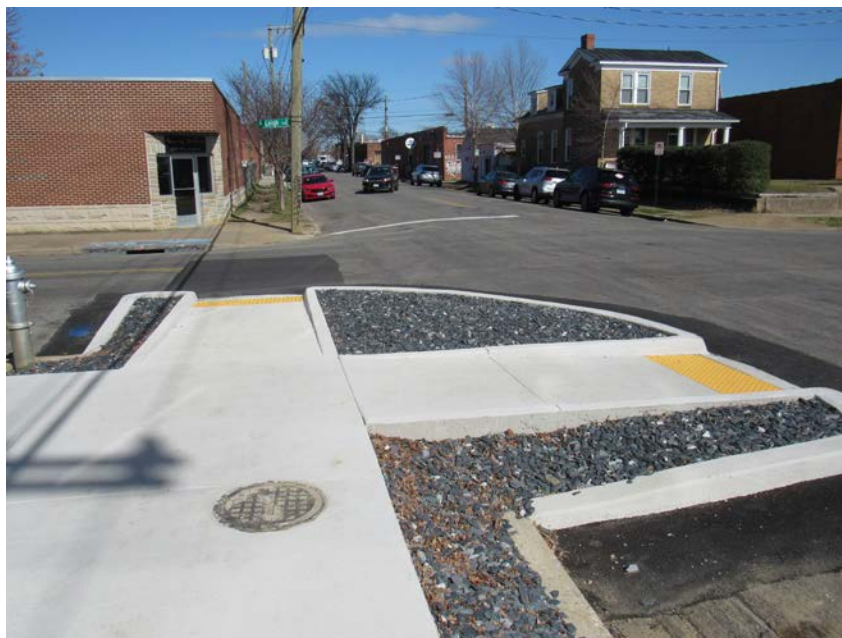
Figure 4-11: Curb ramps with tight corner radius in Richmond, Virginia
