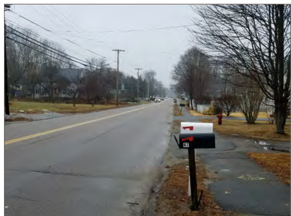
Figure 8: Older sidewalk on South Worcester Street with deteriorated walk surface.
