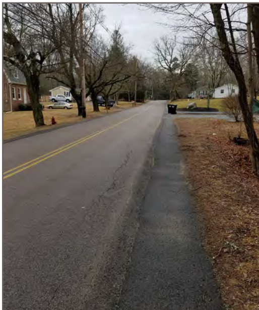
Figure 2: An older sidewalk on Dean Street in need of repair.
