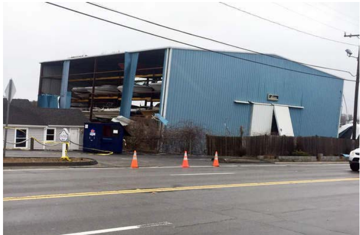
Figure 4: Boat storage facility on Cranberry Highway suffered irreparable damage from the March 2018 Storms.
